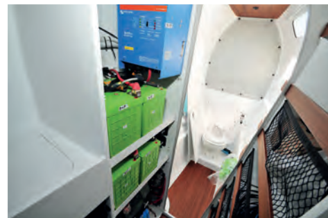
The 14-kWh lithium battery bank is installed aft of the heads compartment to optimize weight centering.
